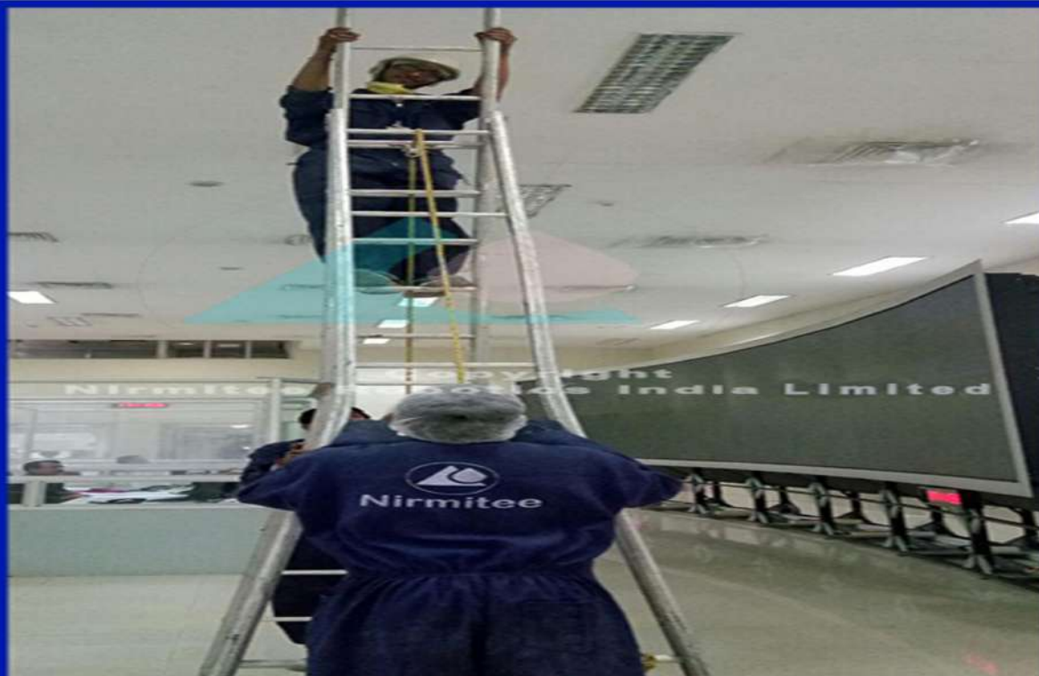
Our Speciality Critical Server and Projection Rooms
